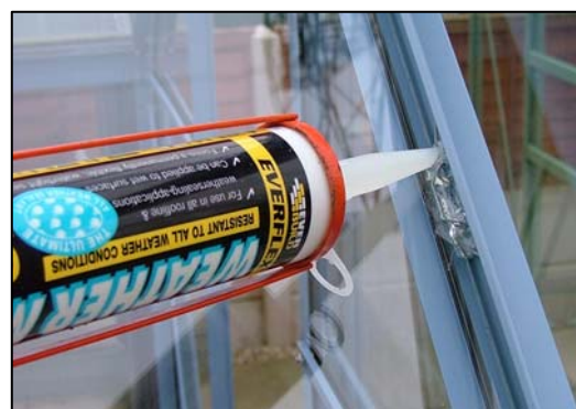
Silicone the glazing clips in to help prevent losing panes in high winds.
