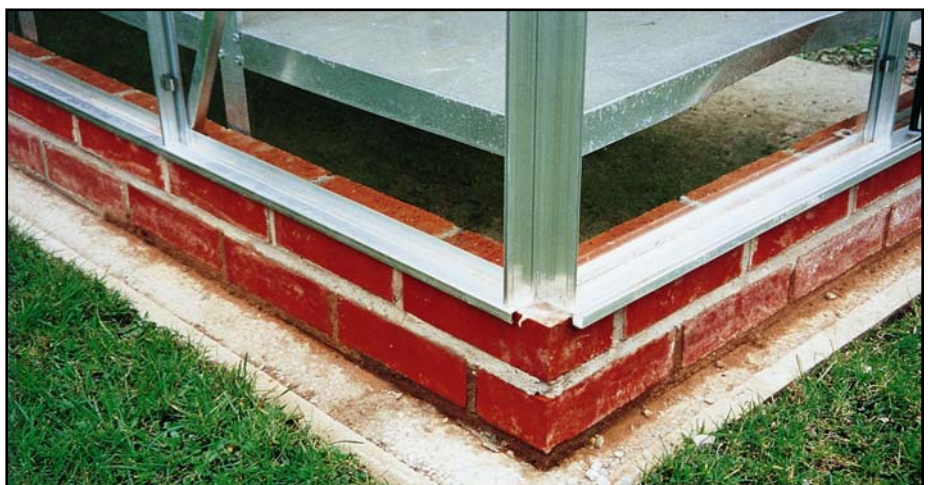
A brick base must be made to the exact millimetre stipulated by the manufacturers base sizes because the cill overlaps the brick.
